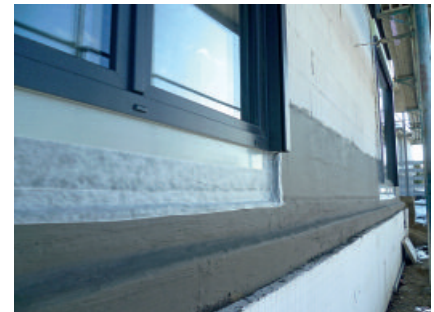
Transition area of floor-to-ceiling window to foundation wall with PCI Barraseal Turbo and PCI Pecithene fleece tape.
