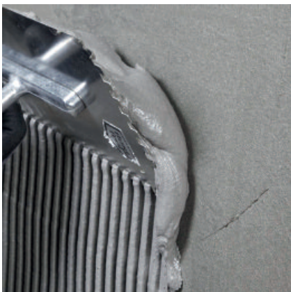
A minimum of 2 layers of PCI Barraseal Turbo must be applied. The material can be applied by notched trowel and smoothed for better coverage control.
