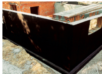
Waterproofing structures in contact with the ground against soil moisture and non-standing seepage water.
