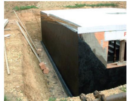
Waterproofing an external concrete basement wall with PCI Pecimor 2K. Good workability due to polystyrene filling.
