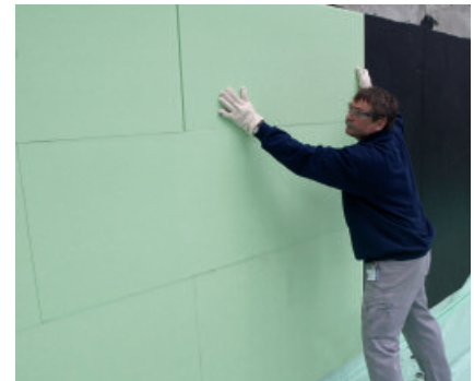
The styrofoam perimeter insulation boards are pressed into the adhesive bed of PCI Pecimor DK.
