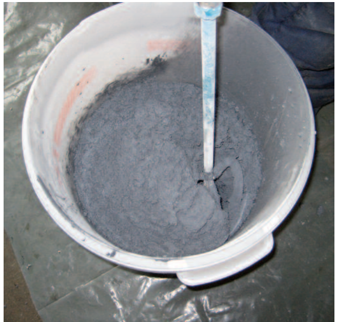
Transfer mixed material to another container to avoid mixing errors at the edges of the pail. Remix if necessary.
