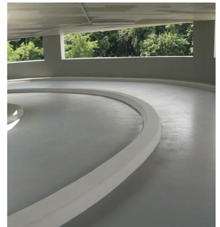
Areas exposed to heavy use of any de-icing agents (salts), e.g. parking decks
