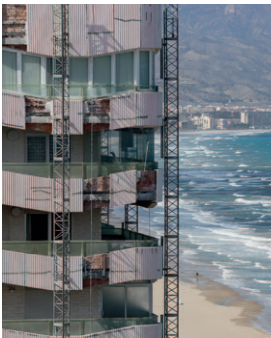
Principle 1: Protection against ingress of chlorides Torres Blancas, Alicante, Spain; Protection with Corrosion Inhibitor MasterProtect 8000 CI
