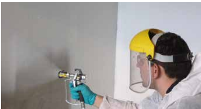
Spray-application of MasterProtect 330 EL as crack-bridging anti-carbonation protection of a car park wall.
